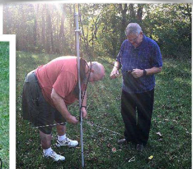
Erik Brom, WBØNIU, left, and Keith Laken, KEØIJI, install a digipeater.
