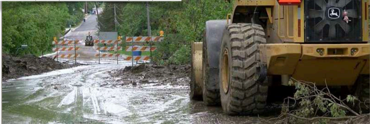
THE VILLAGE OF HOMER SUFFERED DAMAGE IN THE MAY 19 STORM.
